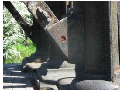
Lost bolt head from bracing connection
