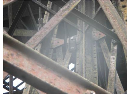
Missing bolt and loose brace
